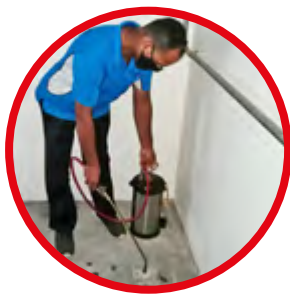
Inspecting pump rooms to remove and treat all potential breeding grounds with insecticide
